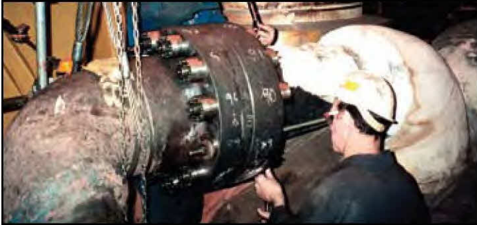
High pressure steam lead with rotational misalignment of bolt holes. Solved leakage and history of bolt failures.
