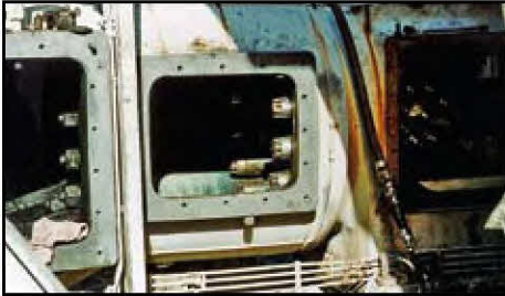
Reciprocating compressor, distance piece.
