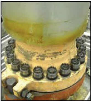
Main steam inlet flange.
