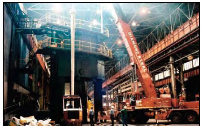
The worlds largest Torquebolt® being installed on a large hydraulic forging press.
