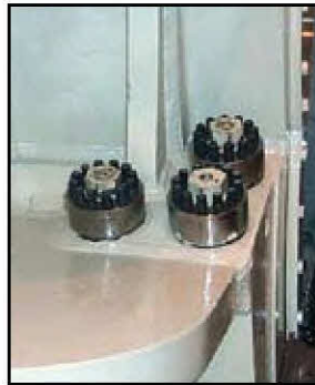
Nuclear plant turbine generator bearing housing. (6) MT-300-8/w Supernuts®.
