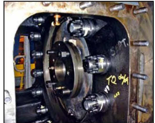
Our products are especially useful in limited space applications, such as this distance piece on a reciprocating compressor.
