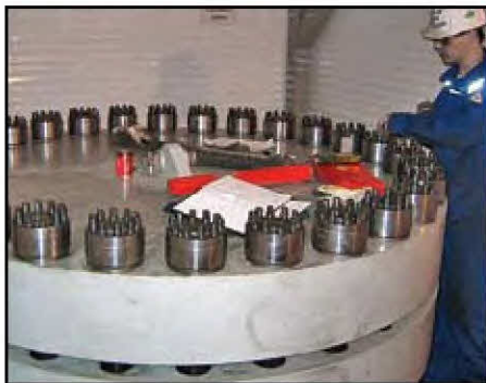
Compressor inlet filter cover.
