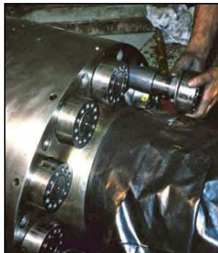
Large turbine/generator coupling. Installation 4 hours, removal 1 hour.
