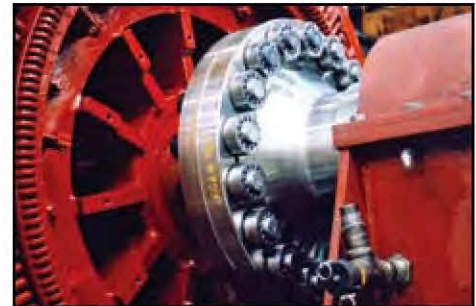
SJX-250-4 on electric motor coupling.
