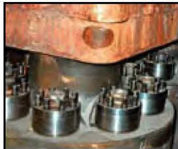
Turbine control valve
