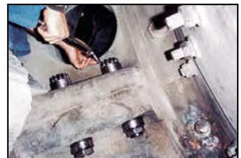
Split Gear segment on rotating kiln
