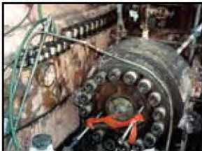
HP turbine and valve
