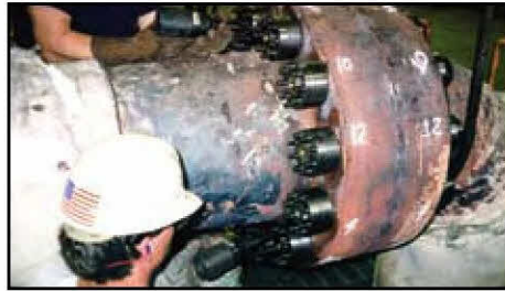
Steam turbine inlet flange. 30 minutes to install, 15 minutes to remove.
