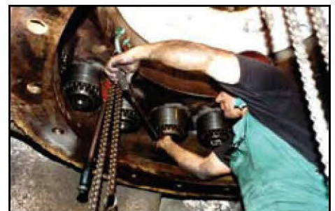
Overhead work is simplified with the low torque requirement on this Turbine Wheel to Shaft bolting. Galling and seizure is eliminated.
